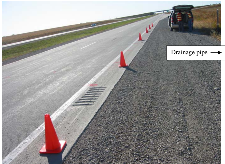
Figure 5.6: Pavement surface distortion, Highway 18 east (mile post 195), Iowa.
